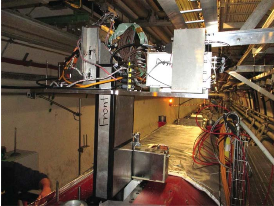
Fig. 9.1: LHCf Arm1 detector and its front-end electronics being installed into the TAN instrumentation slot.
