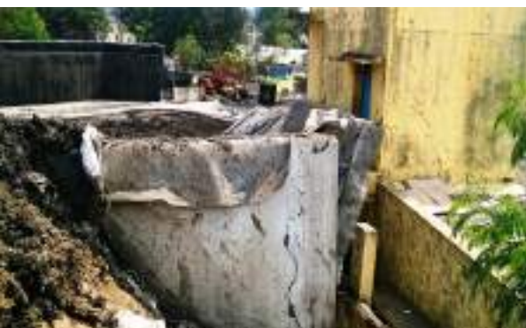
Broken wall-Thinner than the required thickness. Rs. 3.5 crores was sanctioned, but only Rs. 1.25 crore was spent for construction.
