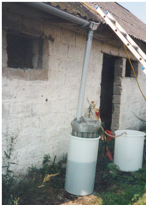
Figure 3.2 Simple set-up for filtration of waste water from roof cleaning in Belarus.
