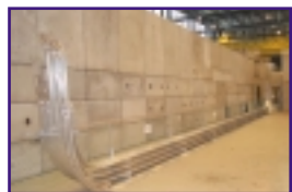
Helium cooling pipes for BT cold mass
