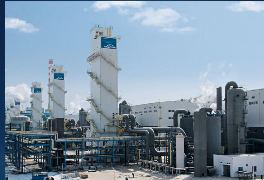
Linde Air Separation Unit
