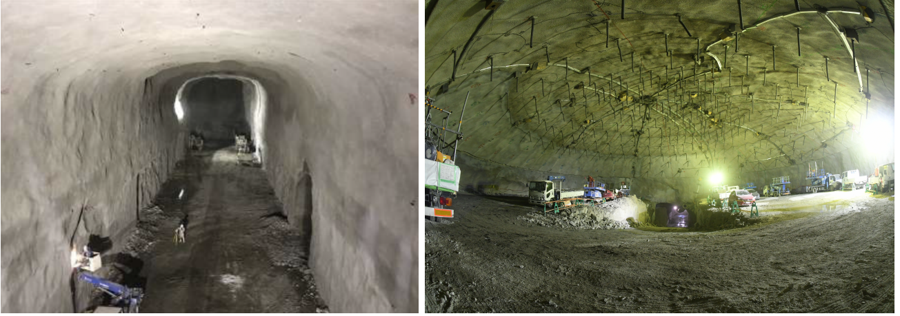
Figure 5: The status of the cavern excavation as of June 2023 is shown, the access tunnel (left) and top part of the dome (right) that will host the Hyper-K water tank.
