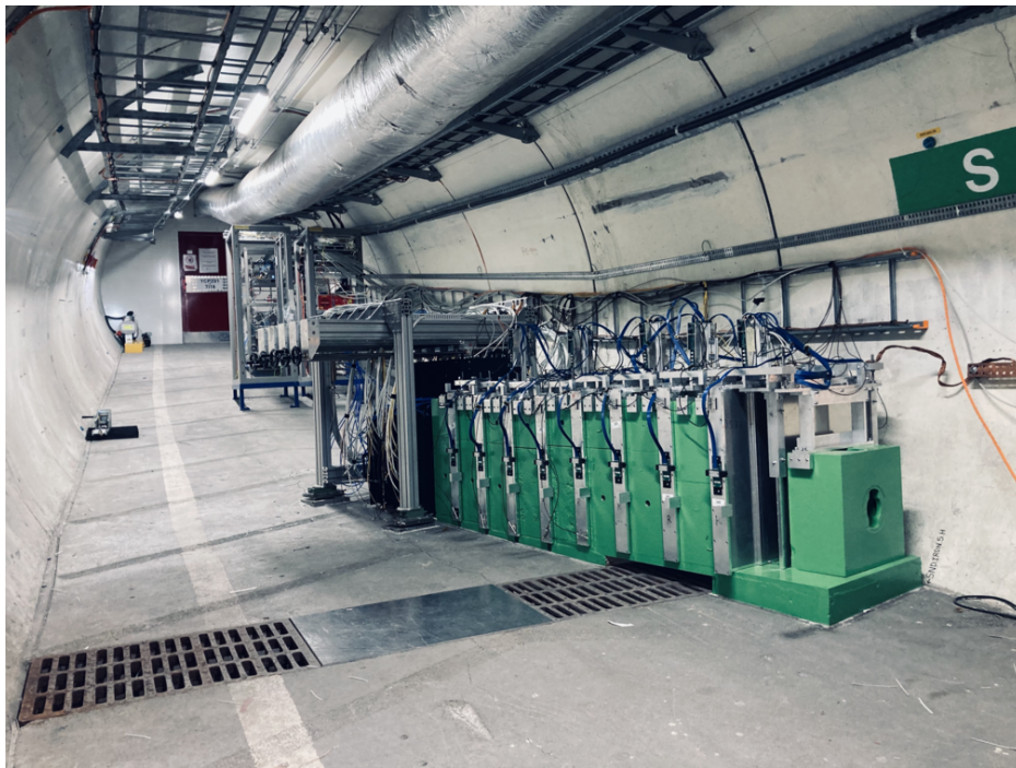
Figure 29. Picture of the installed SND@LHC detector in the TI18 tunnel.
