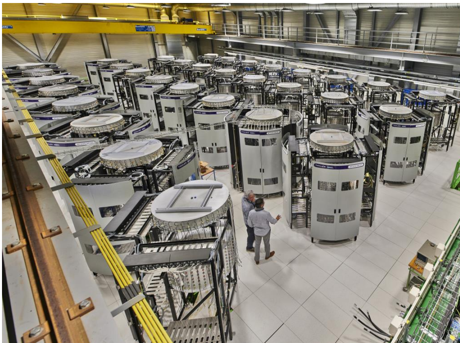
Figure 38. The 32 Thales 144 kW SSPA towers on the mezzanine in BAF3.
