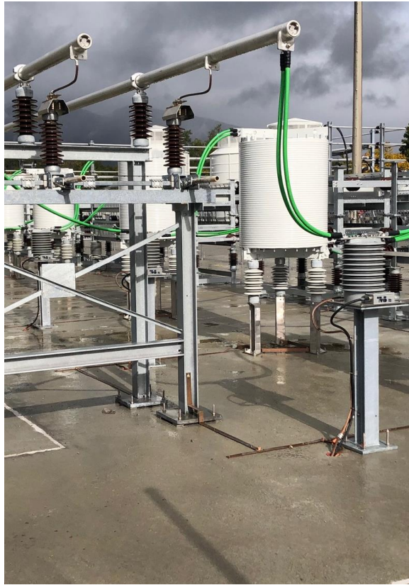
Figure 89. The integration of the IEC-104 protocol in UNICOS is presently used for the communication with the ABB server of the new Static Var Compensators BEQ1 (SPS) y MEQ59 (PS complex).
