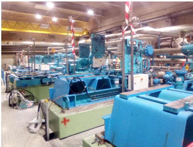
Figure 6. Cryo compressor station at Point 8 (QSCA).
