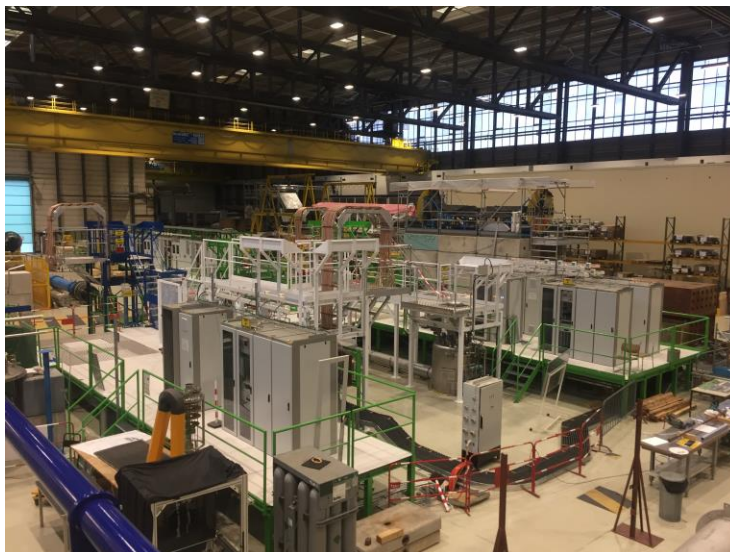
Figure 101: FAIR installation magnet test bench installation.
