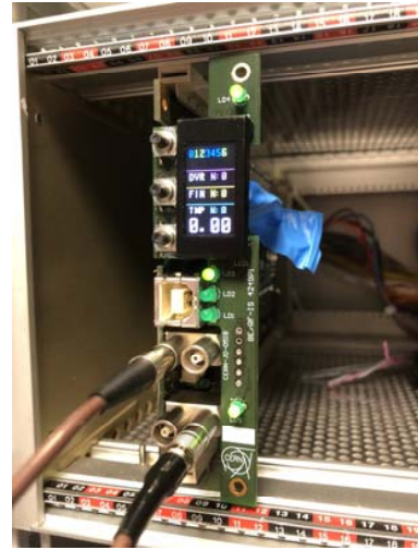
Fig. 23. A compact gate bias controller developed for the PS booster new RF system.
