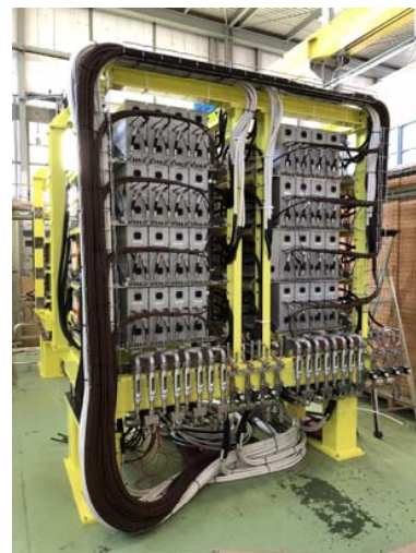
Fig. 1. CERN PSB Cavities and Solid-State Amplifiers before installation.
