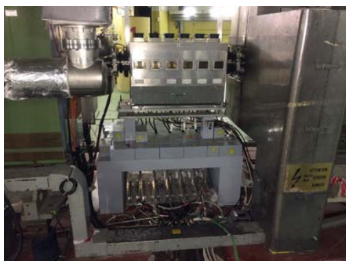
Fig. 2. CERN PS Longitudinal Damper Cavity with Iron Shielding underneath for Solid State Amplifiers
