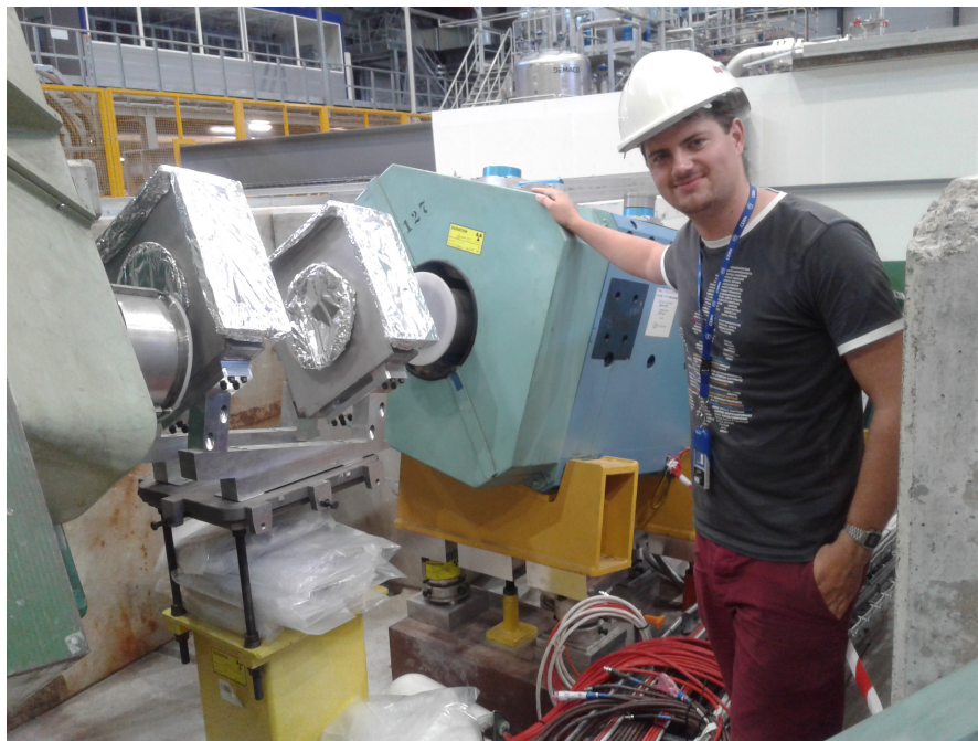
Figure 5.4 – Inspection of the XBPF installation slots BPROF2, BPROF3 (covered by silver foil) in front of the Q24 focusing magnet of the EHN1 tertiary beam line with the author.
