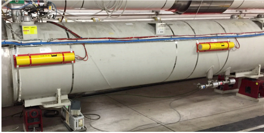
Figure 12: Installed ionisation chamber beam loss monitors (icBLM), yellow cylinders, outside a superconducting quadrupole magnet cryostat. With about 3600 installed icBLMs the beam losses are closely monitored along the LHC.
