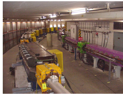
Figure 6.3.: Picture of the view inside the DESY II tunnel [35]
