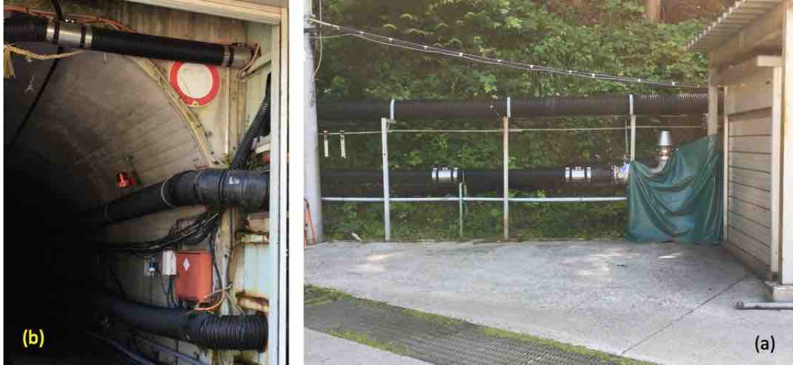
Figure 3.5: Air lines for KamLAND (lower) and SuperK (upper), (a) near pump buildings, and (b) entering mine access road.
