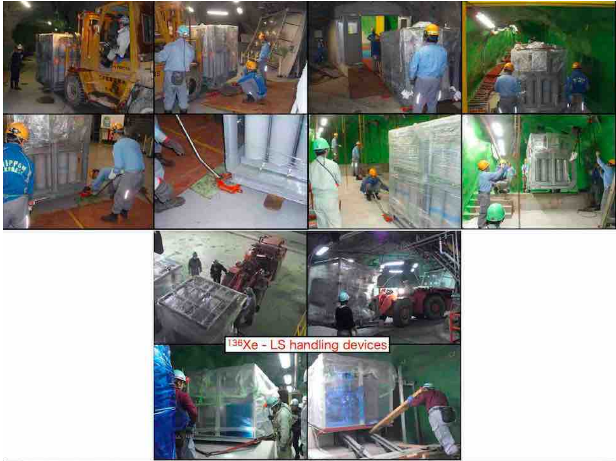
Figure 2.13: Photos from installation of the xenon systems for the Zen experiment. Note the diversity of rigging equipment employed, from forklifts to hydraulic lifters. In particular, note the use of ceiling hooks (second row right side).
