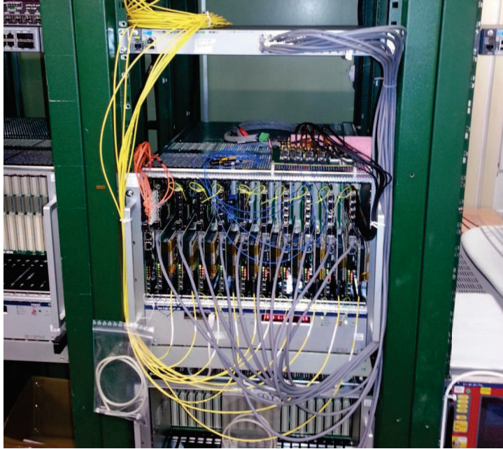
Figure 4.7: VME crate with first 10 GTK-RO boards installed in Bldg. 918’s PC Farm room at the end of October 2014.
