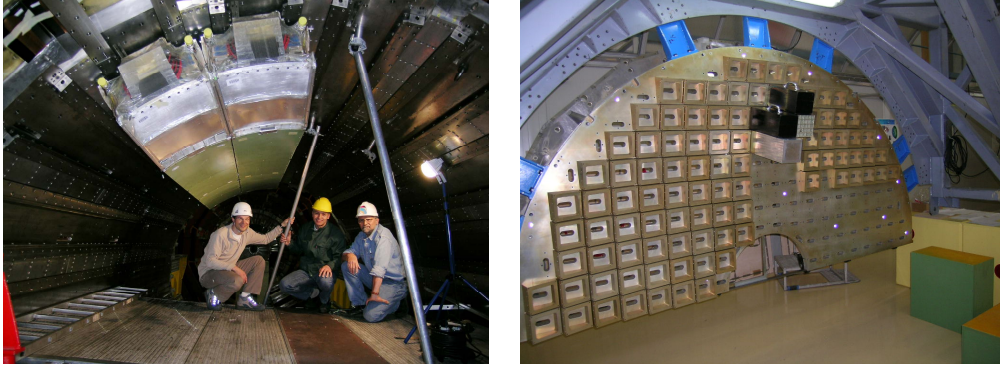
Figure 2.8: Left: Two ECAL barrel supermodules, installed for the MTCC. Right: The 60 mm thick aluminium backplate of an ECAL endcap Dee held on its assembly and installation frame. Four mock supercrystals ( 5 \times 5 crystals) are shown attached in the spacer.
