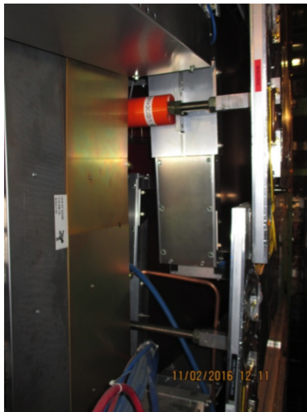
Figure 5.31: Picture showing the available space for RPC services between the CSC and RE4 chambers.
