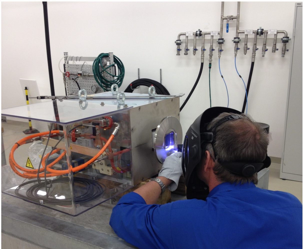
Figure 3.48. Installation of vacuum chamber February 2014
