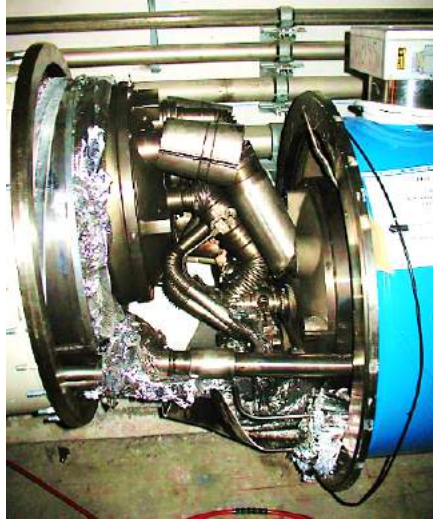
Figure 2.4.: 2008 incident [14]. An electrical fault occurred in an interconnect between two superconducting magnets in the LHC. The photo is taken after the incident. Large amounts of energy were accidentally released and caused severe damage such as displacement of the superconducting magnets as shown in the picture.
