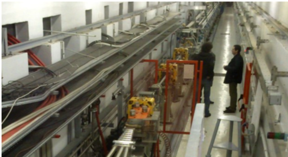
Figure 3.11: View of the LINAC tunnel from the three-way switch-yard, with the two pulsed magnets driving the beam towards the BTF line (3°, yellow dipole, more precisely a modified quadrupole) and the spectrometer line (6°, orange dipole), towards the LINAC (top of the picture). In between, a \approx 15 m drift, with four quadrupoles (yellow). In the upper part of the picture, the passageways towards the parallel modulator tunnel for cables, pipes and waveguides, is visible.
