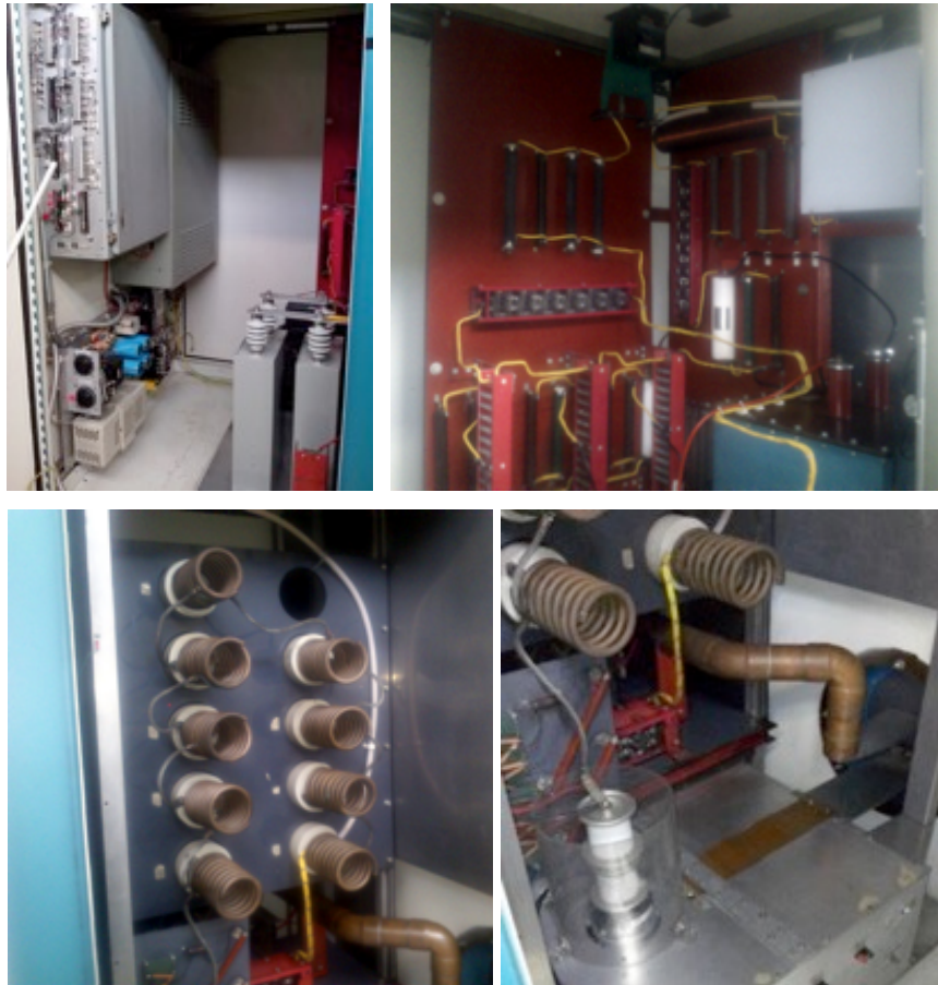
Figure 3.3: The SCR rectifier, the core bias and filament power supplies are placed inside one door of the modulator racks (top left), together with the diode arrays, the large charge capacitor and filters of the charging circuit (top right). In the other rack door: the 9 LC cells PFN (bottom left), the Hydrogen gas thyatron and the conductor towards the pulse transformer (bottom right).
