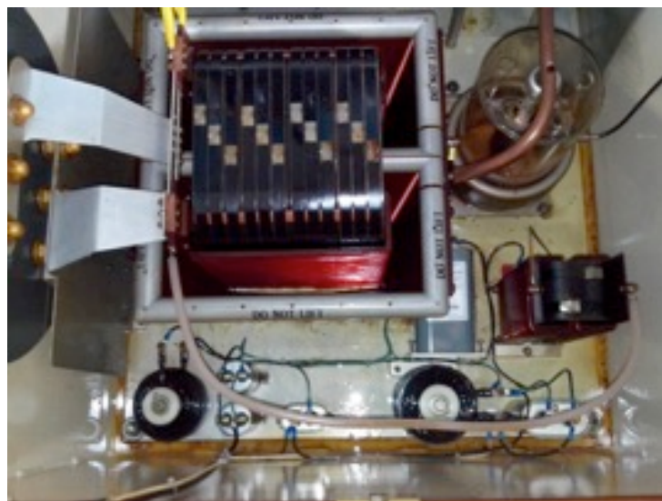
Figure 3.4: The klystron tank, hosting the pulse transformer and the capacitive divider 10,000:1 (for the measurement of the input klystron potential, V_k , on the top right of the picture).
