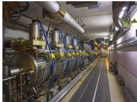
(b) The RF cryomodules installed at IR4.
