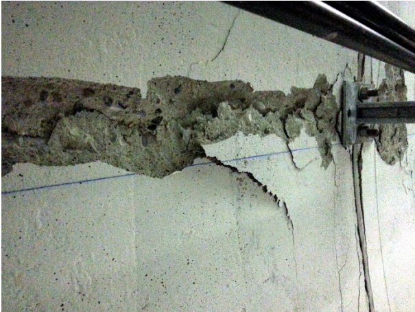
Figure 7: TT10 compression crack on the tunnel crown
