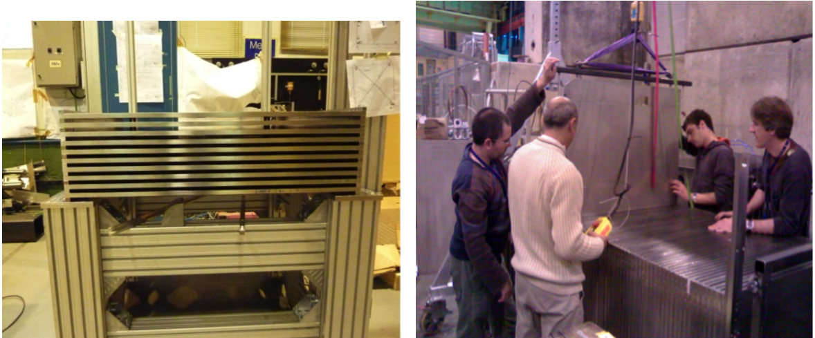
Figure 41: Left: Construction of the self-supporting mechanical structure. Right: Insertion of the cassettes inside the mechanical structure at CERN.
