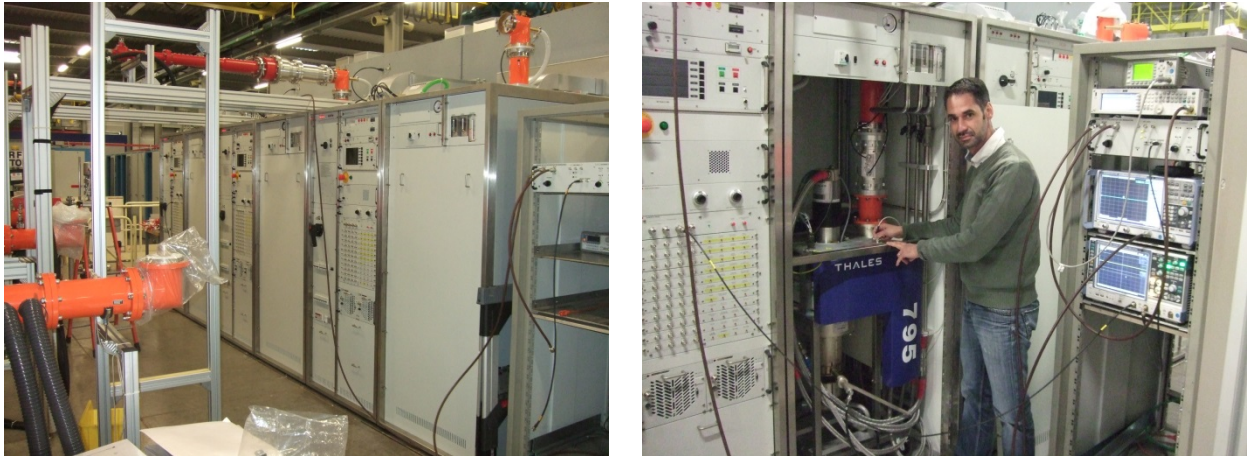
Figure 19: The new, IOT based amplifiers of the SPS TWC800 system during commissioning
