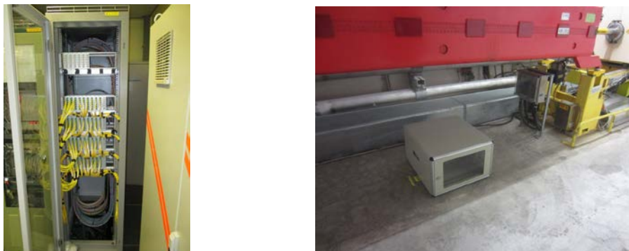
Figure 23: Infrastructure for the new SPS Orbit System. Optical fiber distribution rack (left). Mini-chassis to house the radiation hard front-end electronics underneath an SPS dipole (right).
