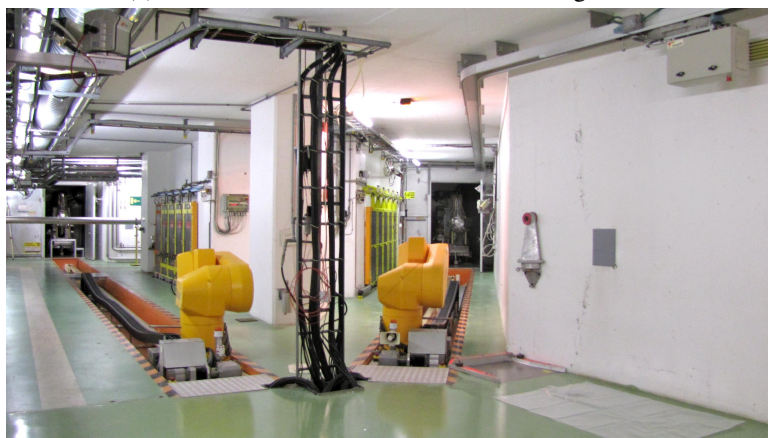
(b) A view of the ISOLDE target area showing the KUKA industrial robots for handling radiation targets.
