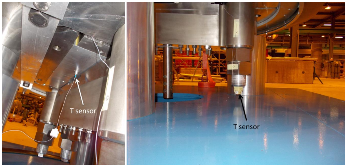
Fig. 9.8.6 – Temperature sensors at the bottom of the magnet structure: dummy and rod.
