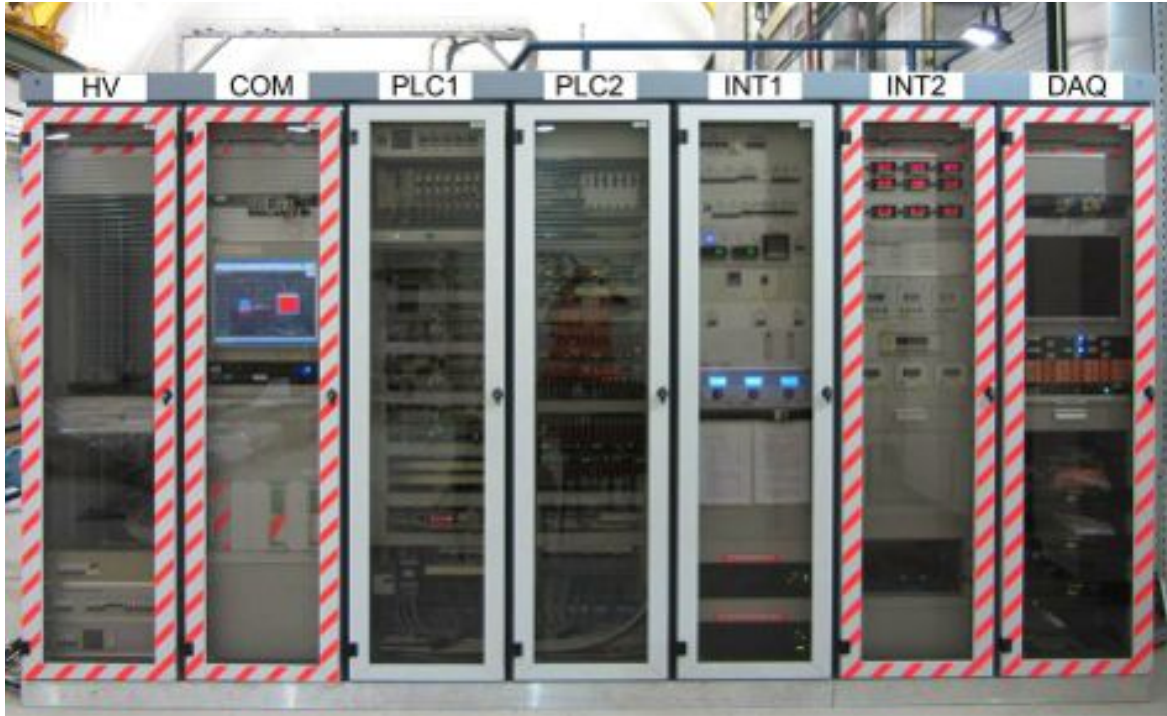
FIG. 110: The seven standard 19 racks containing the ArDM (CERN RE18) control system (COM, PLC1, PLC2, INT1 and INT2 rack), the high voltage supply of the PMTs (HV rack) and the data acquisition system (DAQ rack). The system was built in Collaboration with the CERN/PH-DT group.
