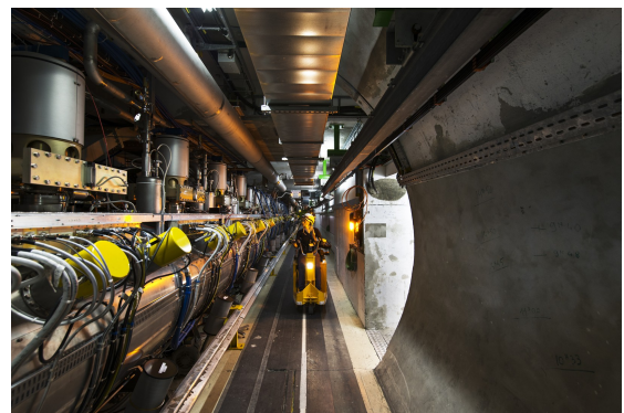
Figure 8: LHC superconducting cavities (in the machine tunnel) [2]
