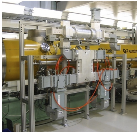
(a) A two-feed unit of PDS1, incorporating a VTO and H-hybrid, installed on a cryomodule at NML.
