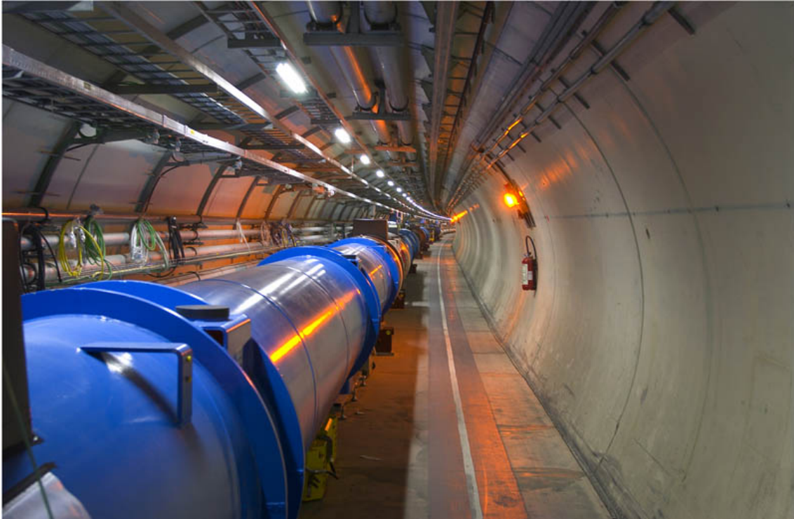
Figure 1.2: View of the LHC tunnel with already installed parts of the accelerator ring [10].
