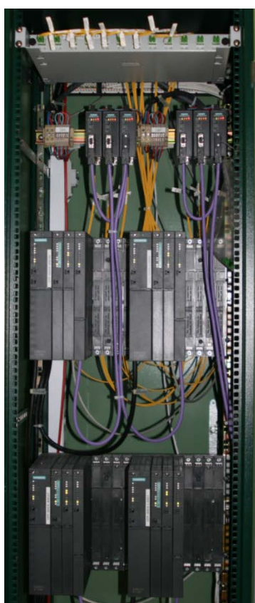
Fig. 6. Rack with 4 PLCs for 2 sectors (1 cryogenics site)
