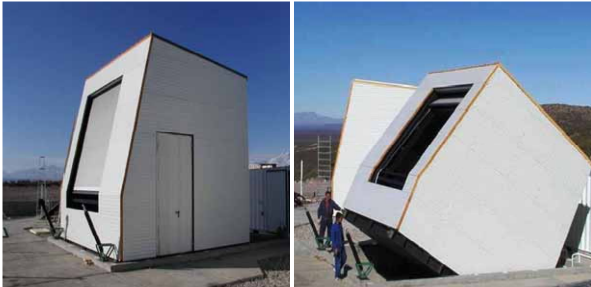
Figure 166 – A single HEAT fluorescence telescope under construction in horizontal ('down') position (left) and tilted ('up') position (right) [171].
