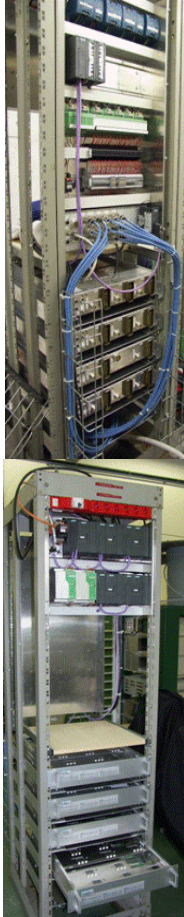
Figure 3. Rack with electronics for on/off (PV, QV) and analog (CV) valves for QRL (back and front side).
