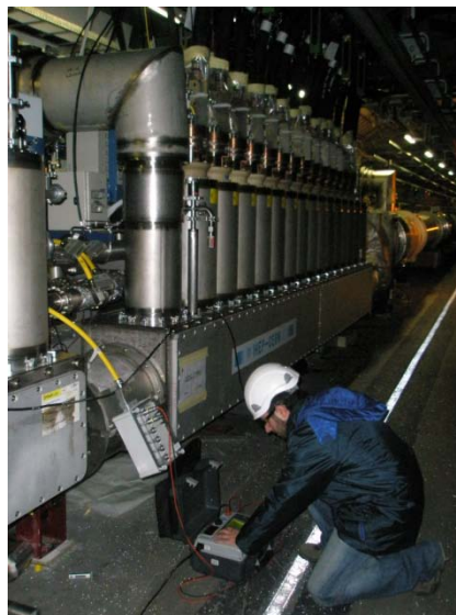
Figure 10. High Voltage tests in one of the 52 DFBs of various types.
