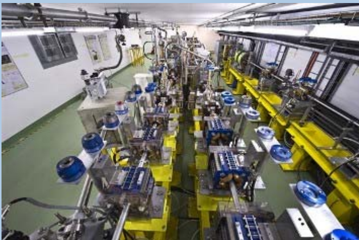
The Two-beam Test Stand (TBTS) of the CLIC Test Facility (CTF3). Image courtesy of Maximilien Brice, CERN.
