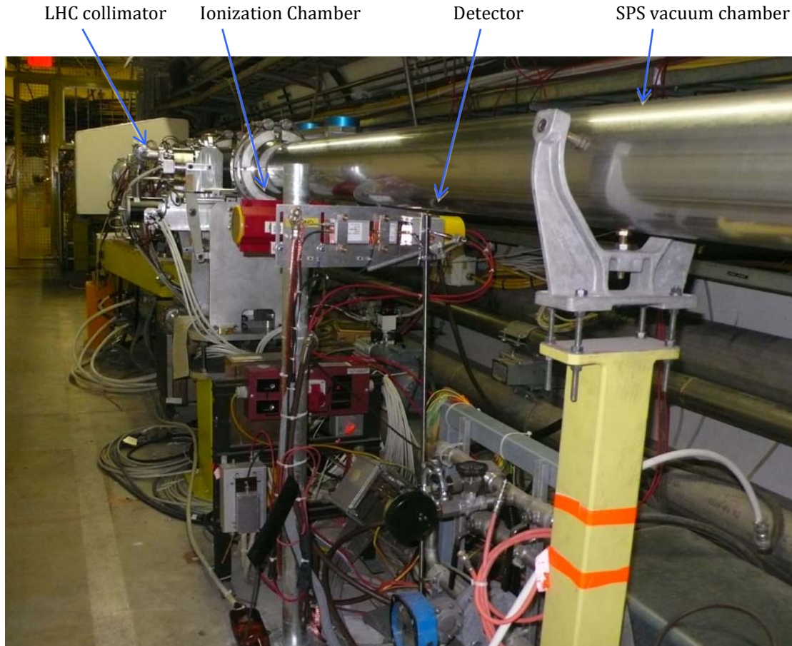
Figure 4: The detector is installed in BA5 directly below the beam vacuum chamber and about 2 m downstream of the LHC collimator.
