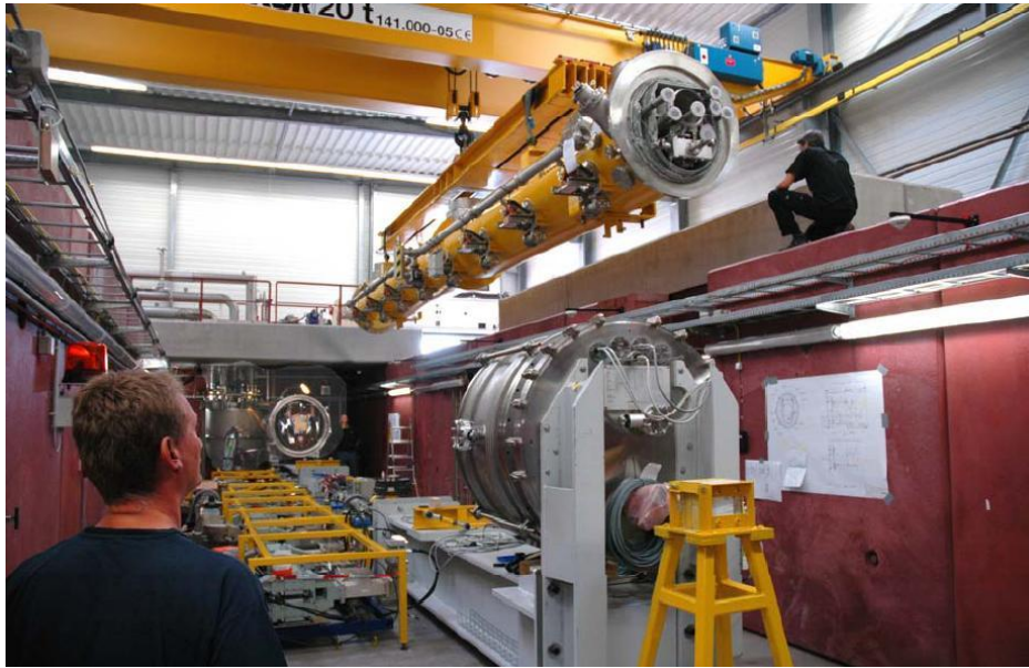
Fig. 1.7 – FLASH module #6 (ACC6) during installation in the CMTB facility
