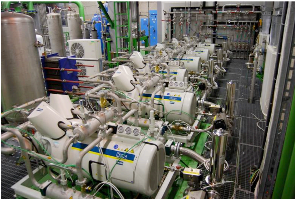
Figure 6. Evaporative system main plant in USA15. Four compressors are visible (white housing)
