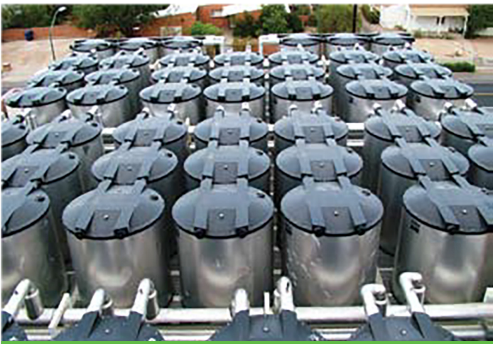
Ice storage integrated with CHP provides 23,400 ton-hours of cooling at the University of Arizona in Tucson. 4 Photo courtesy of CALMAC
