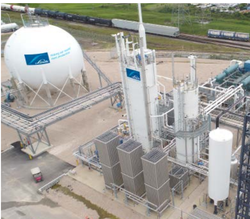
Linde's LaPorte, TX hydrogen production and liquifaction plant
