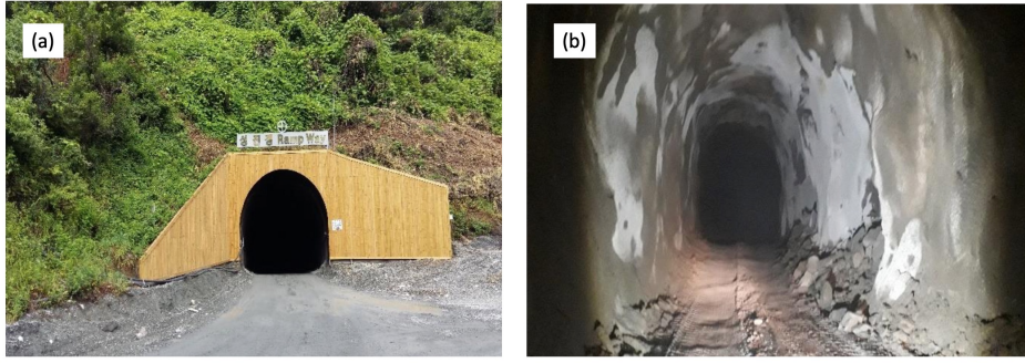
Figure 3.4: Photos of the Handuk Iron Ore Mine ramp. (a) the adit, entrance way, (b) internal ramp section. Nominal cross section is 5 \times 5 meters, but is highly variable along the 6.6 km length. Most important is that the mining trucks can pass through.
