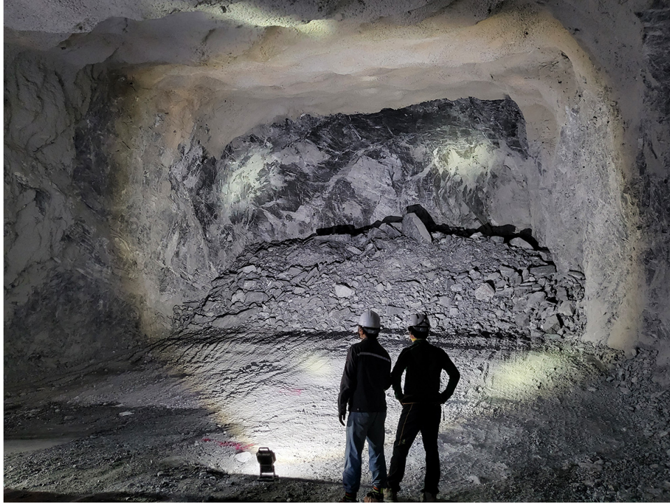
Figure 2.3: Photograph taken December 16, 2021 showing the status of the cyclotron room. Blasting is almost complete.
