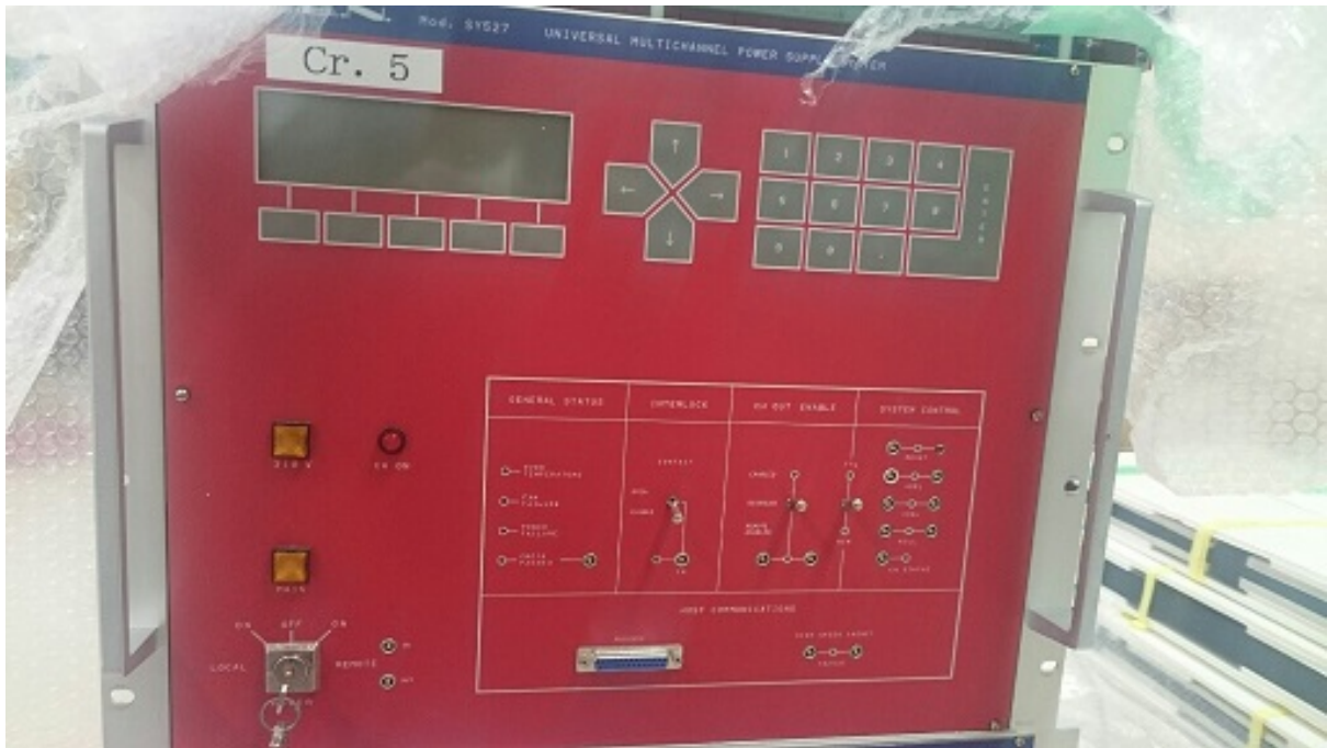
Figure 42: Photo of SY527, CAEN mainframe.
