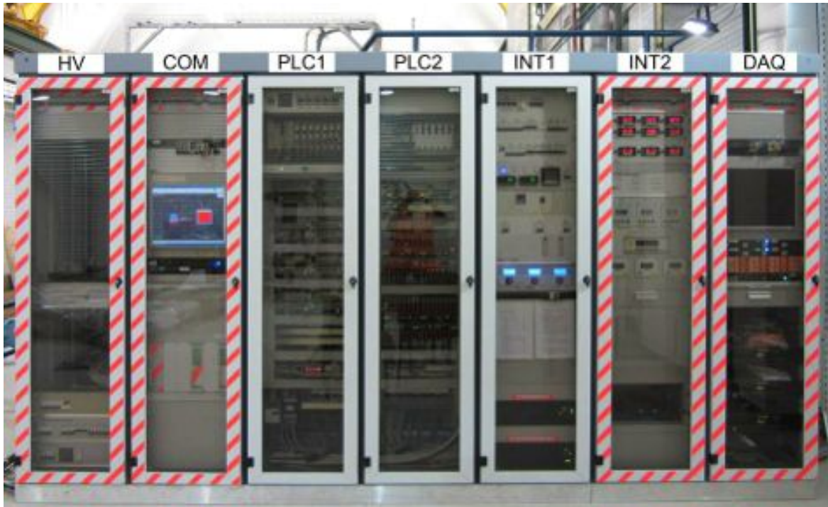
FIG. 110: The seven standard 19 racks containing the ArDM (CERN RE18) control system (COM, PLC1, PLC2, INT1 and INT2 rack), the high voltage supply of the PMTs (HV rack) and the data acquisition system (DAQ rack). The system was built in Collaboration with the CERN/PH-DT group.
