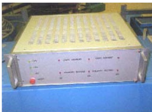
Figure 6: Picture of the white circuit bypass capacitor protection system (main control box)
