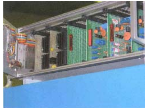
Figure 4: The white circuit bypass capacitor protection system circuit board
