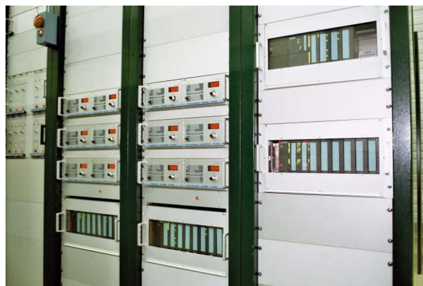
Figure 2: Electronics racks of one high voltage generator showing thyatron heater power supplies, thyatron heater and terminating resistor controllers.
