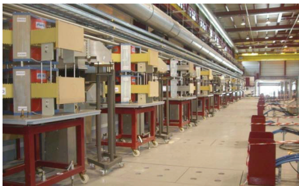
Figure 6: RF Network installed in the Linac4 Hall.
