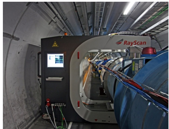
Figure 4: The RayScan Mobile X-ray Tomograph in operation at the LHC.
