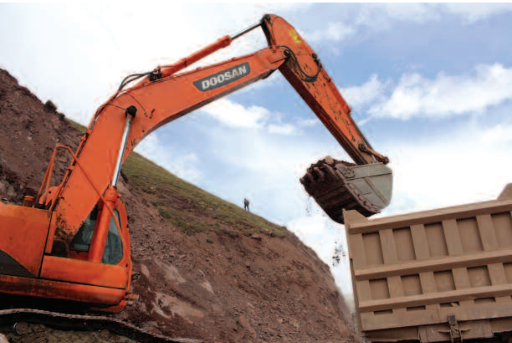
Heavy machinery moves dirt from the side of a mountain, during the construction of a new road in southern Qinghai Province.
