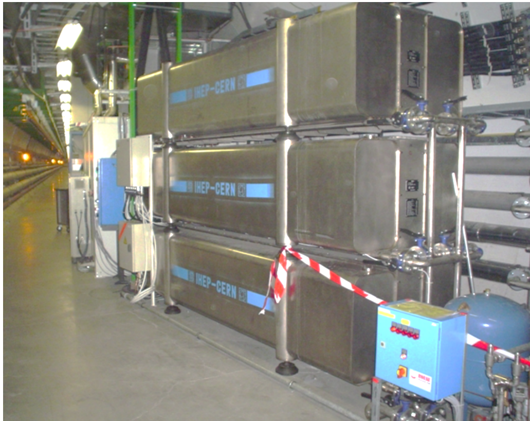
Figure 2.13: Picture of a single dump resistor configuration of a main dipole circuit. Each resistor, consisting of three larger resistors connected in parallel, is built to withstand the full stored circuit energy of 1.3 GJ. Together with a mechanical switch, these resistors comprise the energy extraction system. Photograph courtesy of CERN [56].
