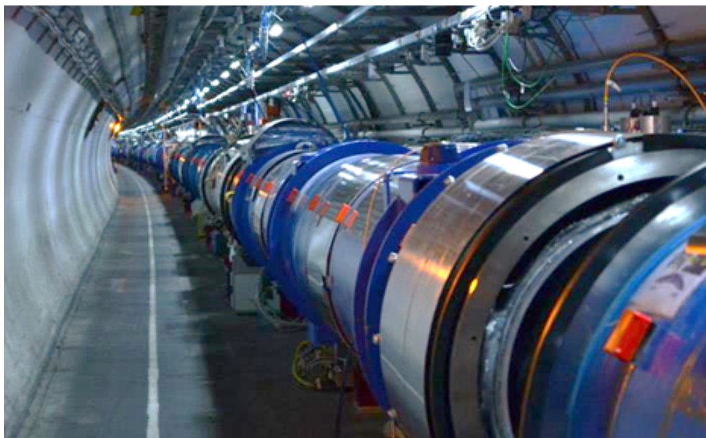
Figure 1.7: Picture of the LHC Arc cryostat which encases, amongst others, the main dipole circuits. Openings can be seen along the cryostat as this picture was taken during a repair campaign (discussed in Chapter 3).
