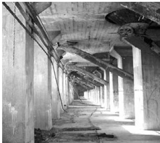
The Concrete Central elevator showing the raised basement, an invention of Harry R. Wait. (Photo by Lynda H. Schneekloth)
