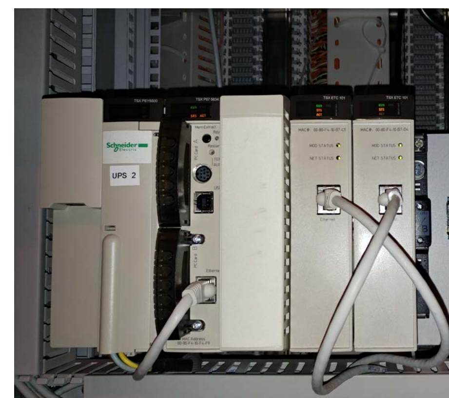
Schneider Electric Premium PLC with 2 EtherNet/IP network cards
